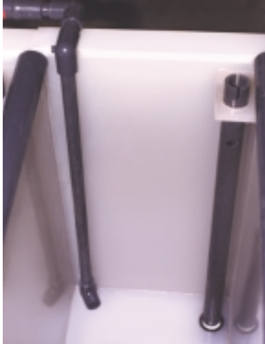
Top view of an overflow rinse tank. The pipe on the left is for the inlet water which is directed diagonally across the bottom of the tank where it is circulated to the top and exits the tank through the overflow pipe which is connected to the common drain pipe. Tanks may also be constructed with a dam type overflow along one side of the tank. It should be noted that the E-Kleen, E-Prep, InstaBlak and E-Tec tanks are not connected to the drain pipe.
